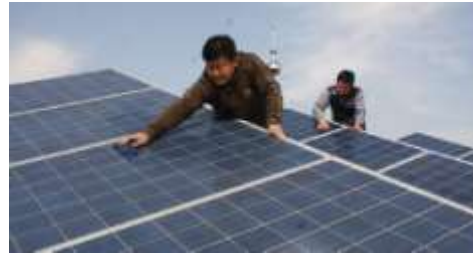
Fig.2. Manual cleaning of photovoltaic cells
